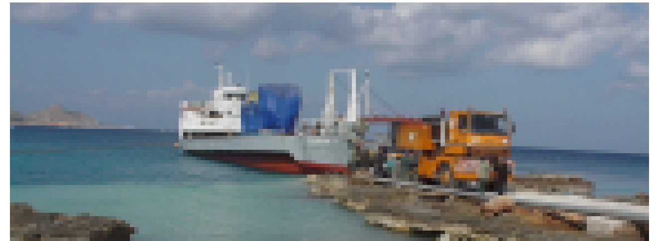
Skidders and 400-tonne mast jacks were used to safely offload a 280-tonne diesel engine from a special ship in March 2000. That time the job site was in the sunny Greek Islands. As usual, the work also included installation of the diesel engine.
